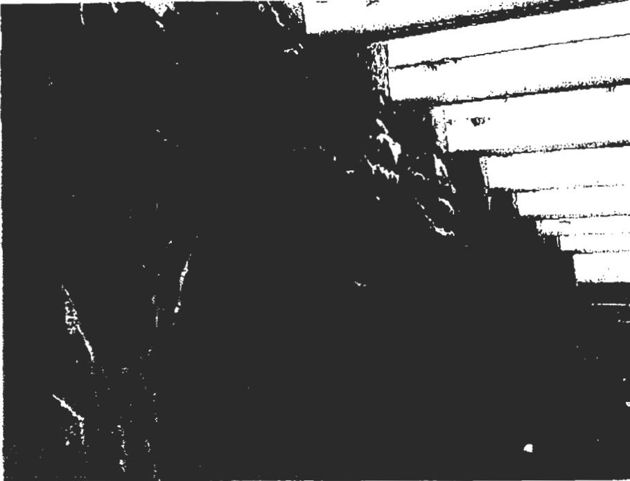
This photo shows the results of Efflorescence
